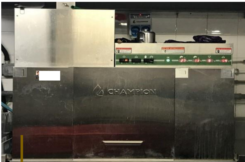
Heat-recovery dishwasher in the kitchen of the Harbour Restaurant
