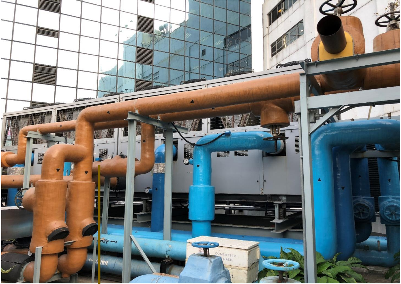
Multi-function heat pump chiller on our roof
