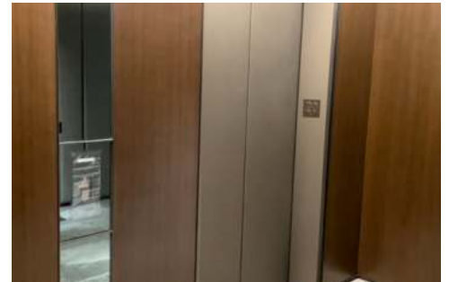
Variable Voltage Variable Frequency (VVVF) Lift Drive System
