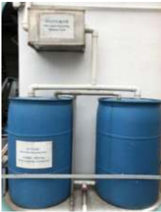
Rainwater Collection System
