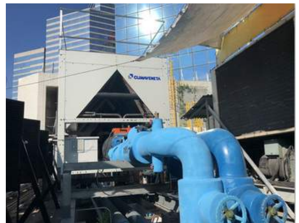
Oil-free Chiller, installed in 2018
