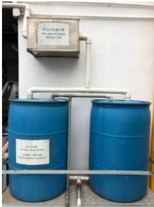
Rainwater Collection System
