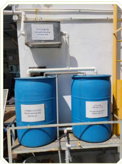
Rainwater Collection System
